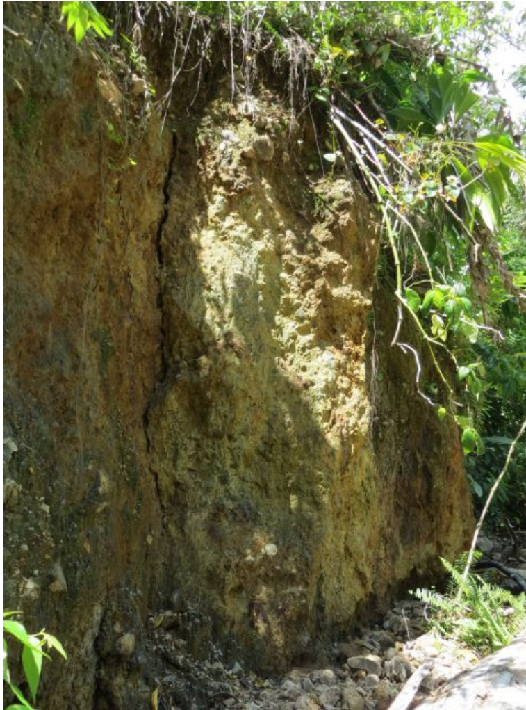
Fig. 2: Near vertical cracks in the steep sided slopes of the Morne Prosper river valley.
